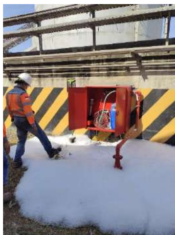
Gambar 3. 7 Inspeksi Hydrant Foam
