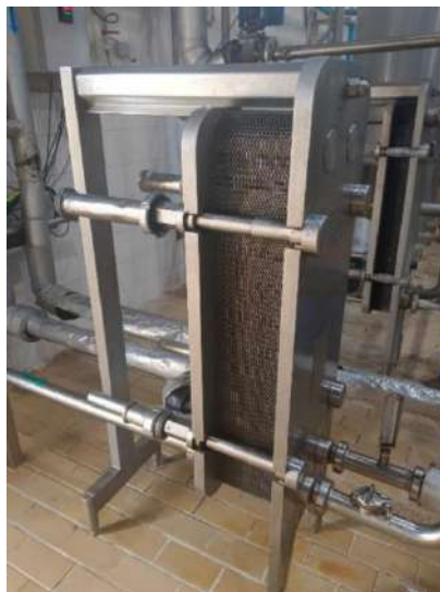
Gambar 24. PHE (Plate Heater Exchanger)
