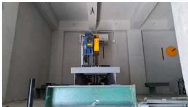
Figure 4. Ruang Mesin Lift
