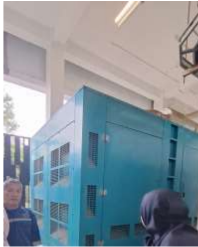
Figure 3. Mesin Genset Listrik
