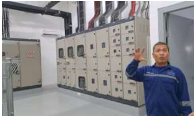
Figure 2. Ruang Energy Panel
